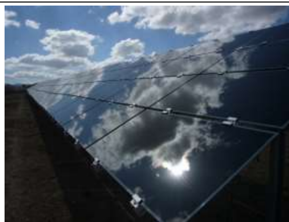
Photo 5-2 Typical PV array
